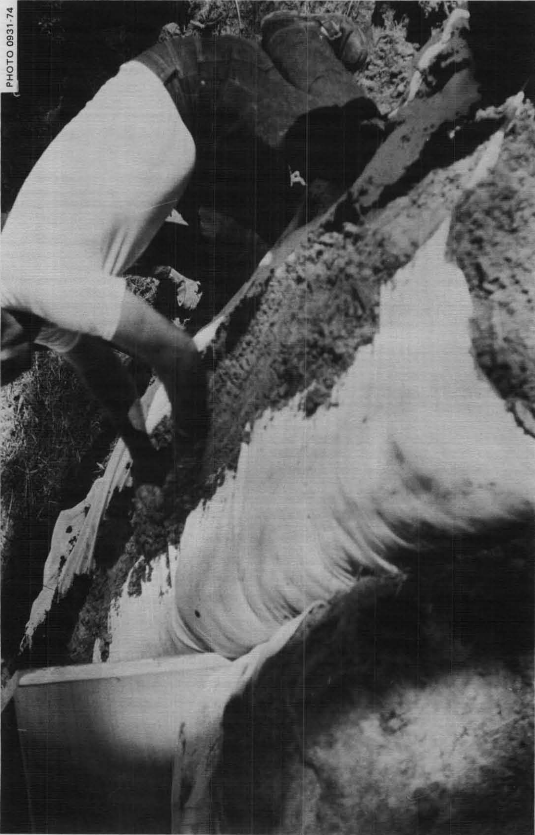
Fig. 5.5. Packing earth into what soon would be the hook of a roll. This photo was taken after the upper, free part of the sheet had been pulled down and over the earth that had been piled on part of the sheet while part of it was supported by the form made of an interior door. A part of this sheet had been folded down into a shallow ditch dug in the mounded earth; this ditch was below the line of packed-in earth on which the father's hands are pressed.
